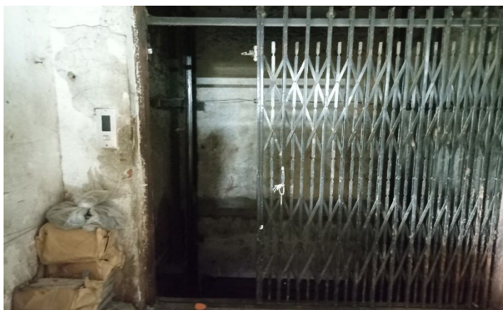
Figure 1: Open door of the lift
