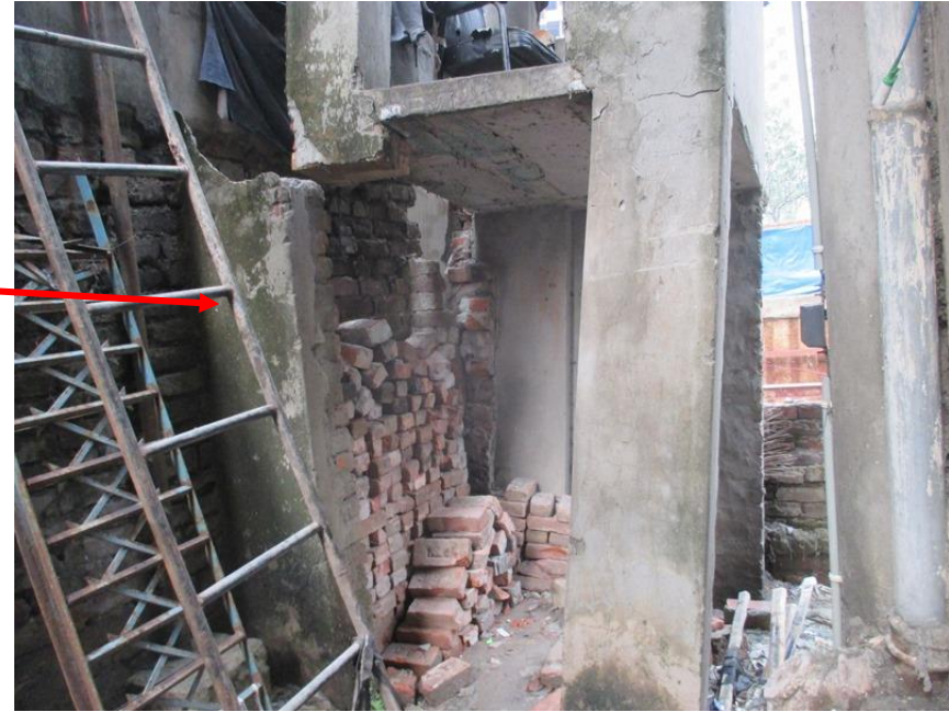
Broken column of the security room
