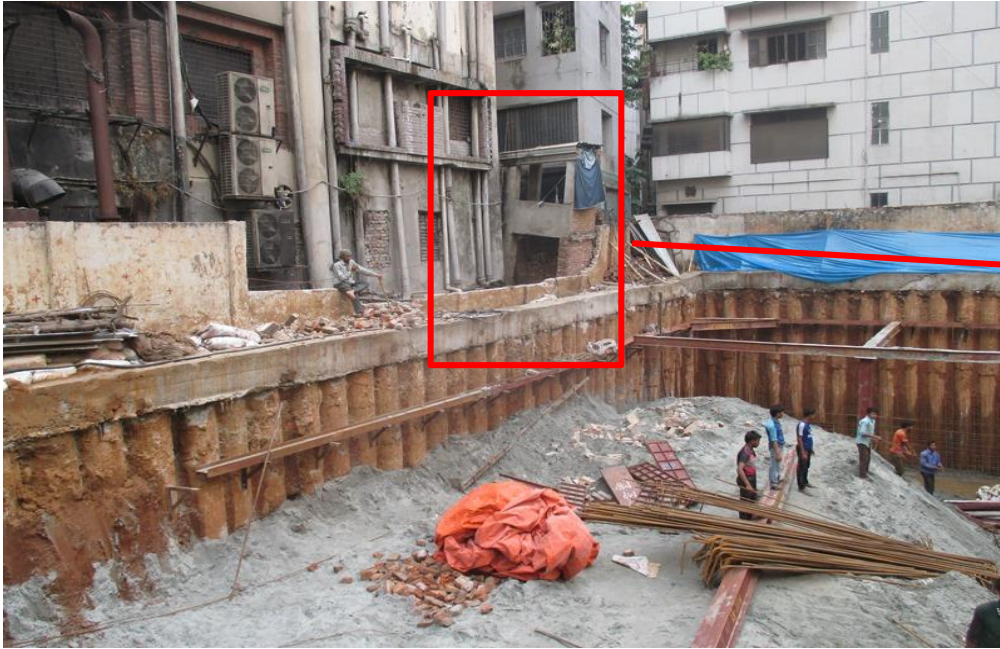
Tilting/partial collapse of security room
