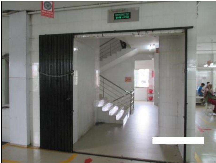
Before: Collapsible gate
