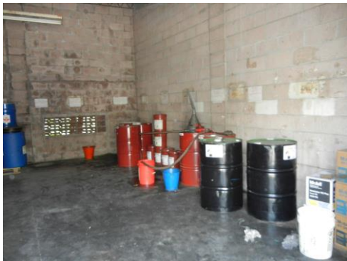
Left: Ungrounded thinner drum in flammable storage room. Note spill on floor.
