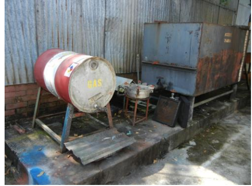
Kerosene drum without secondary containment stored outside.
