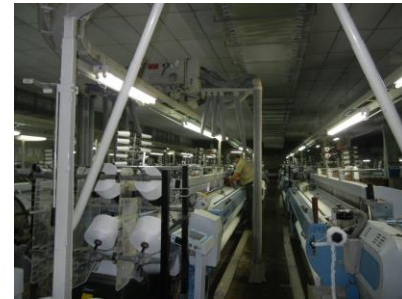
Dust vacuuming system and exhaust duct in weaving area.
